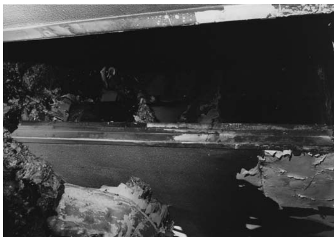
FIG. 2—View of the door leading to the master bedroom—Soot deposit on both side of the doorframe suggesting that the door was open during the fire.
