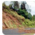
Landslides and Mudslides
