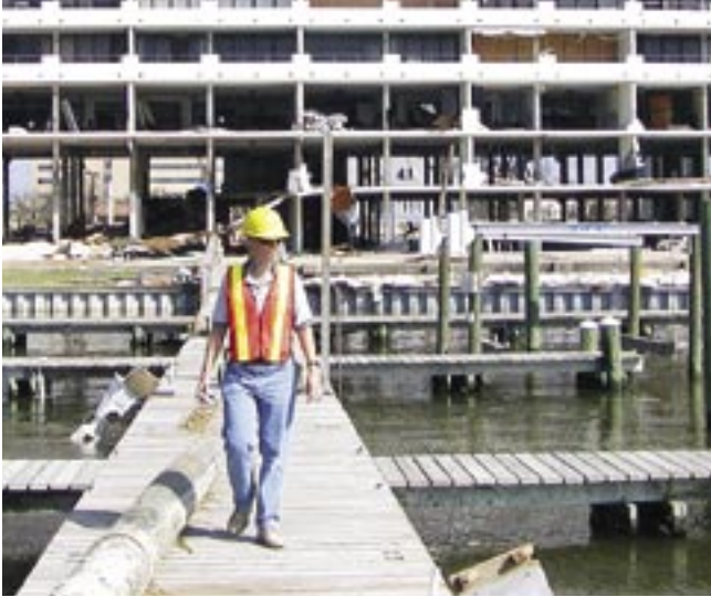
Ronald Riggs discovered a gauge to the height of Katrina's storm surge in Biloxi, Miss., where two floors of the Windjammer Condominiums were blown out and the third sustained major water damage
