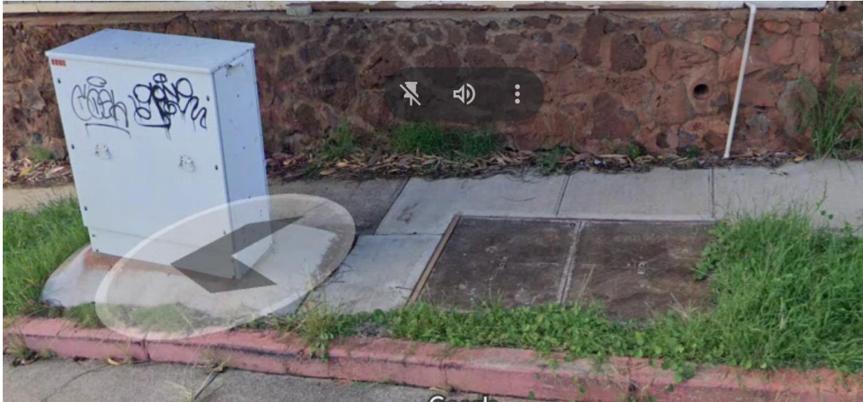
Figure 5: Example of a location where underground broadband is surfaced to a conduit to serve a household
