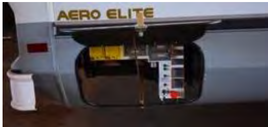
Figure 9. Bus Export Power Unit.
