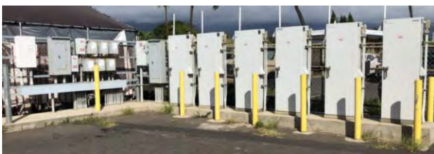
Figure 1. Sunverge SIS BESS + PV units.
