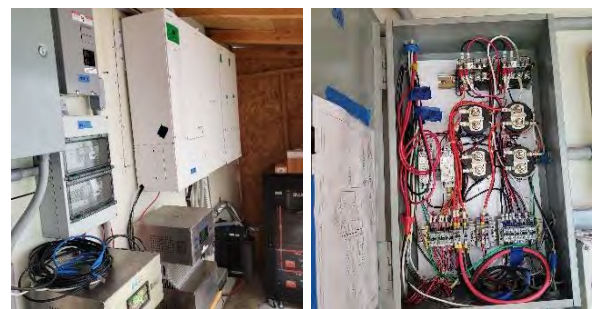
Figure 3. View of project electrical room and one of four control boxes with high voltage switches.
