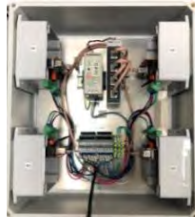
Figure 2. Load measurement box with ARGEMS devices.
